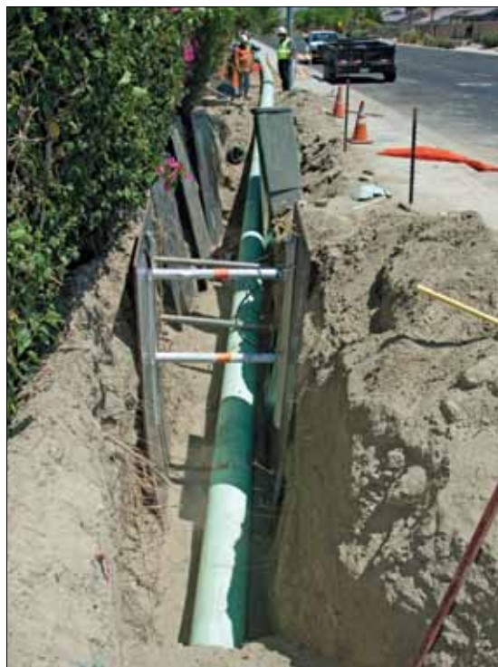
This project was done by Downing Construction and took place near the intersection of Avenue 48 and Shields Road in Indio.
